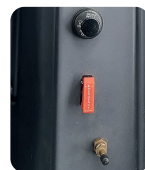
Emergency cut off switch
